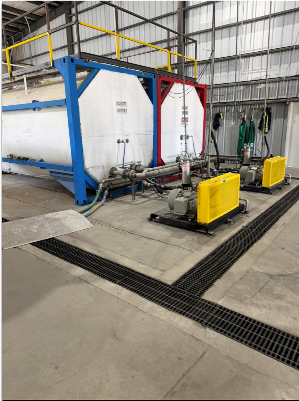
Photo 3 – Tank Wash Area (Rinse Water Tanks)
