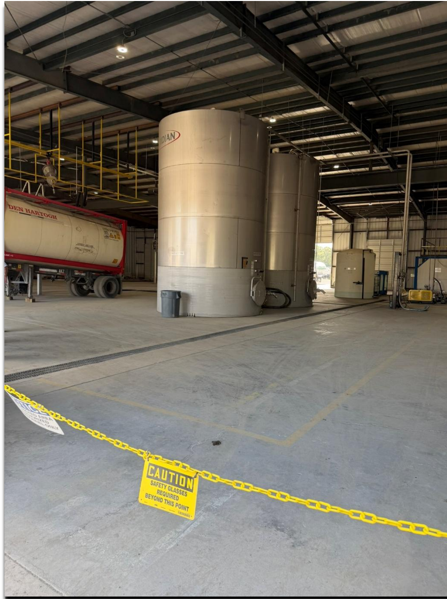
Photo 1 – Tank Wash Area (Storage Tanks)
